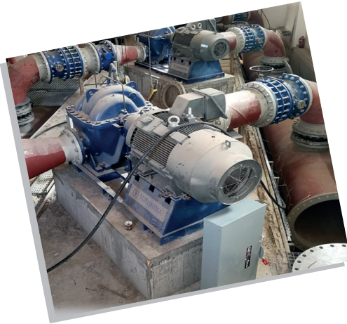
3B Project Pumps
