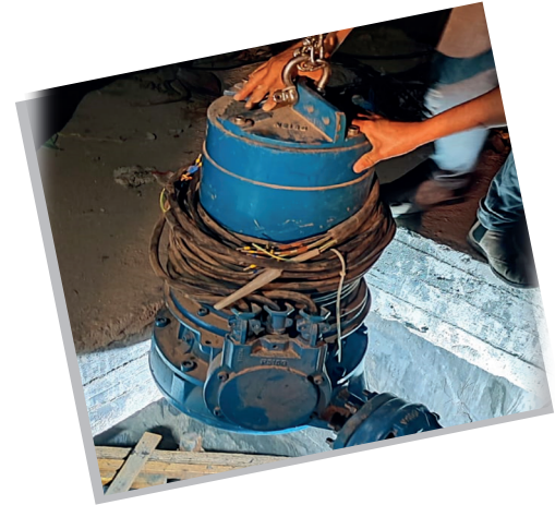
Marina Project Pumps
