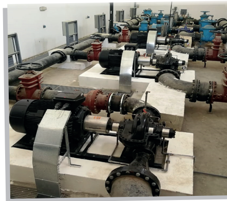
Taif Project Pumps
