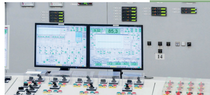
■ Smart Solutions and Control Systems
